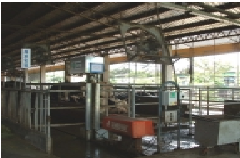
Fig. 4. Computerized controls for fans and a sprinkler cooling system for dairy cattle
